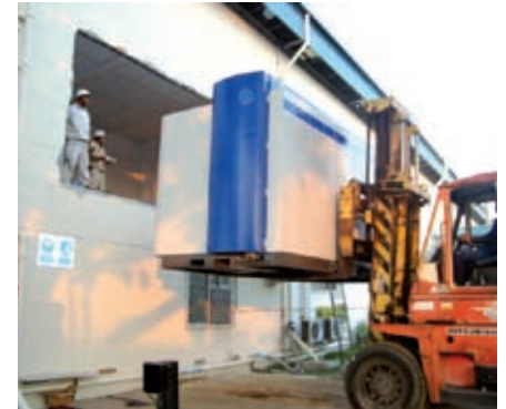
Not even a concrete wall on the first floor was an obstacle for the METAPLAS-DOMINO.
